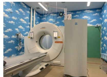
Figure 2: Genano 5250A air purifier in CT room
